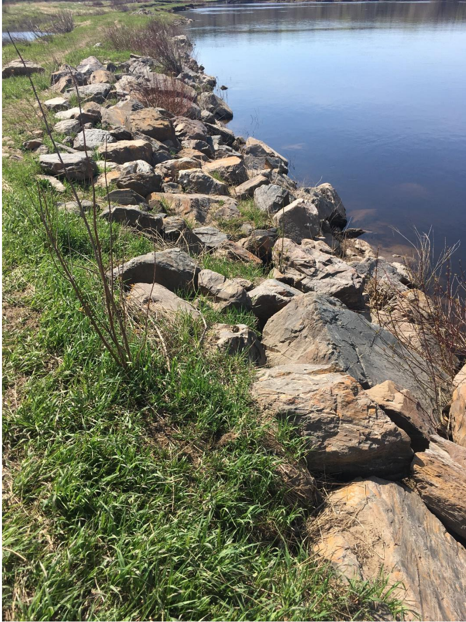
B02b. Rock Armouring. Photo taken post-flooding on May 21, 2020 at 10:44am.
