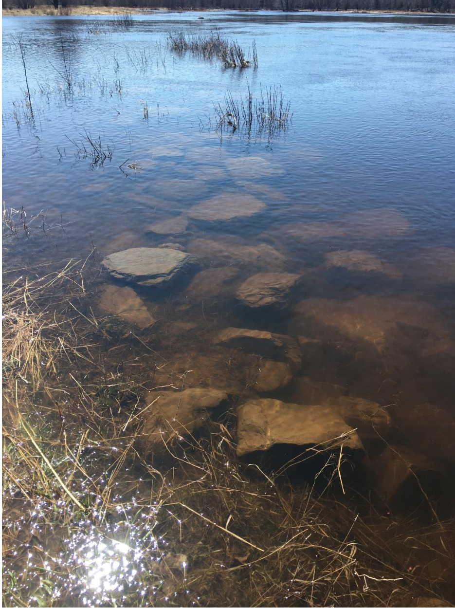
B02a. Rock Armouring. Photo taken during flooding on May 6, 2020 at 11:39am.
